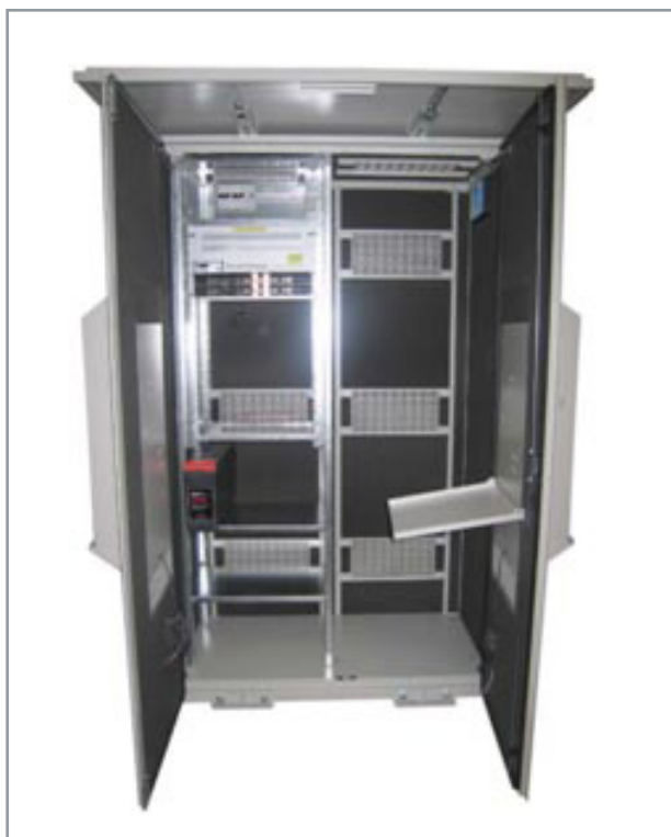
DCEN-02 Internal view
